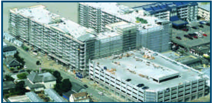
The Reward walls of North America’s largest ICF structure were completed in early August.
