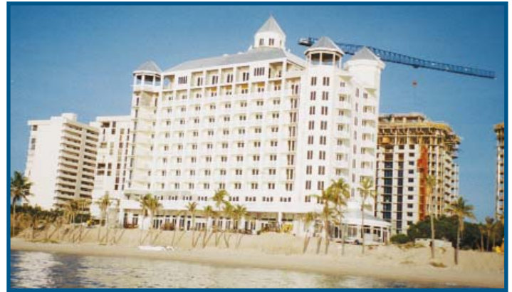
Reward ICF walls and several other innovations help make this Best Western hotel ecologically friendly.
