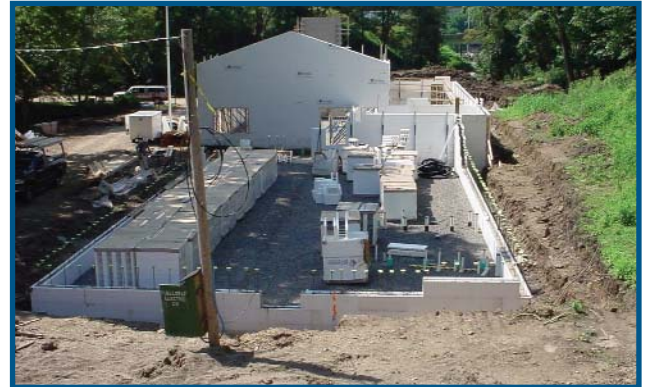
The designers of the Boy Scouts of America's McGinnis Education Center in Pennsylvania, built with Reward walls are working to earn a silver LEED certification for the building.
