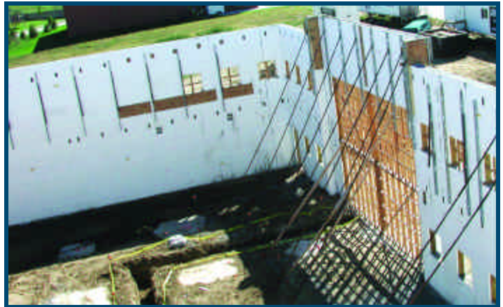
The 24- and 28-foot walls are among the tallest unsupported ICF walls in Nebraska.
